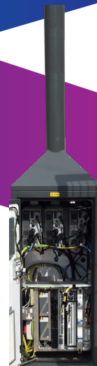
Small cell cabinet
