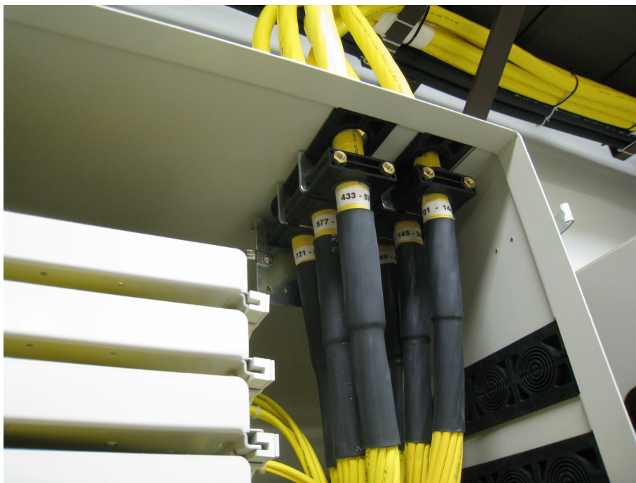
Figure 8. Detail of Top Entry Cables
