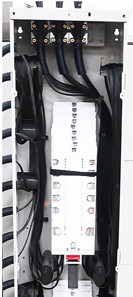
Figure 10. Cable Routing in Splice Cabinet Top Splice Deck
