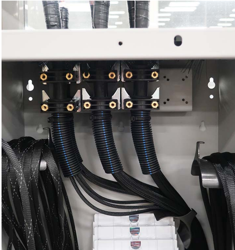
Figure 17. Example of Facility Cable Clamping
