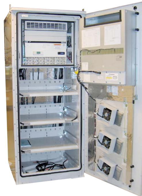
11.22: Integrated cell site power and battery cabinet
