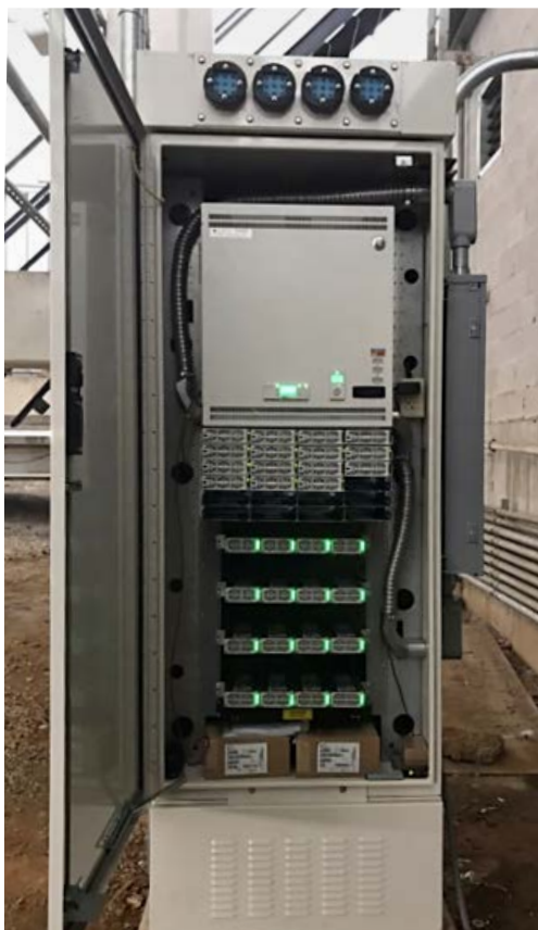
11.28: A PowerShift-loaded distribution cabinet, providing power to a football stadium's DAS remotes
