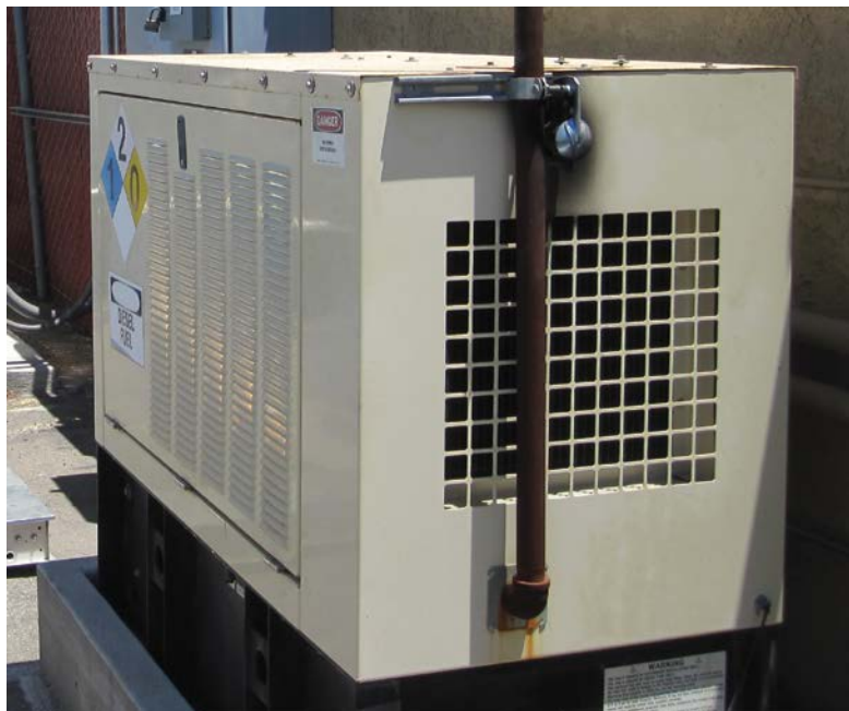
11.6: ac permanent generator
