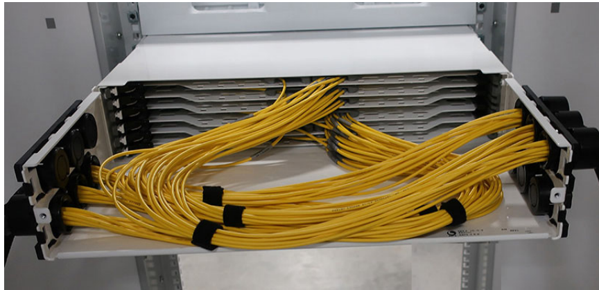
Figure 16. Cable Bundled With Hook-and-Loops
