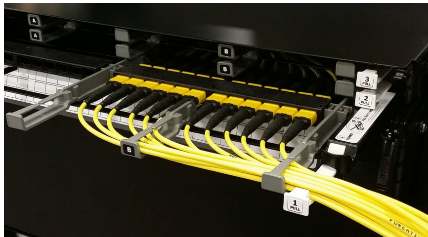
Figure 32. Patch Cord Routing on Front of Panel
