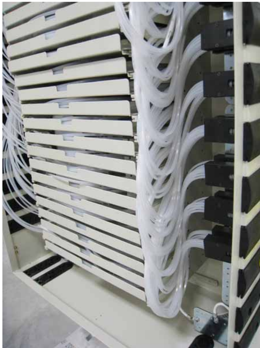
Figure 20. IFC Cable Protective Tube Drip Loops
